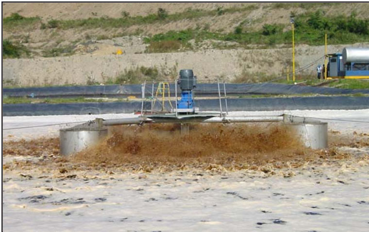
Typical TWISTER™ Low Speed Aerator on floats.
