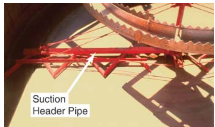
Common header pipe removes sludge in Type DR design.
