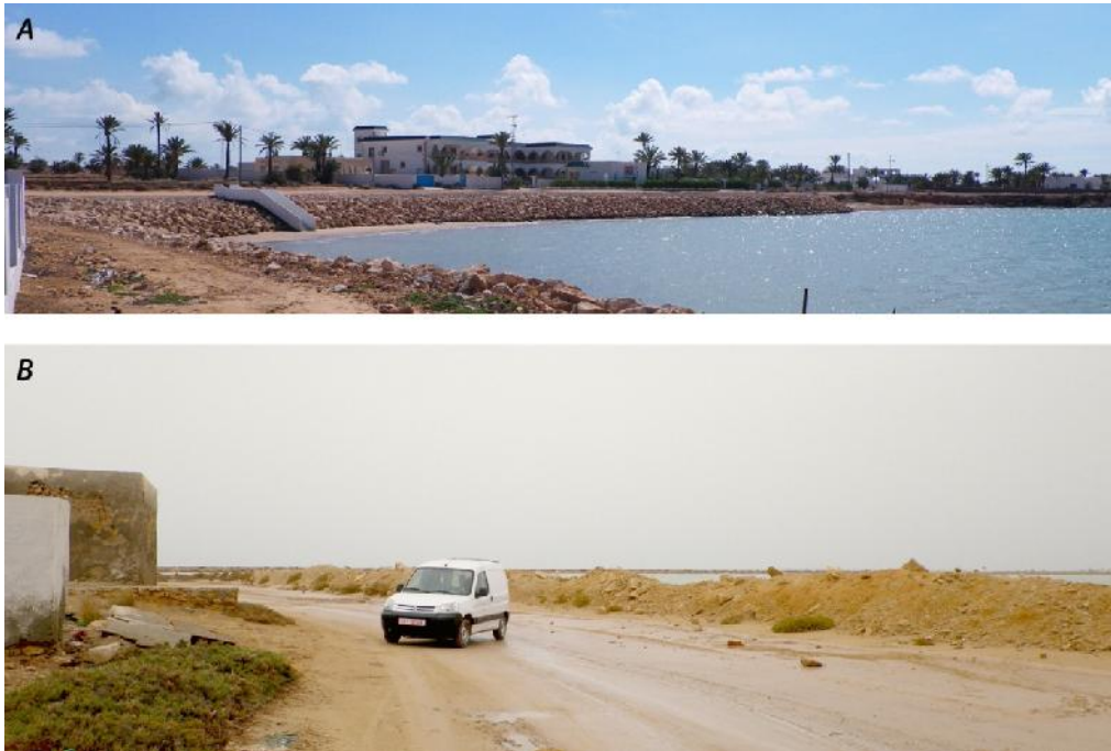
Fig. 4: A. Photography of the state rock fills in March 2010). B. Photography of an individual sea wall just after a storm in March 2009.
